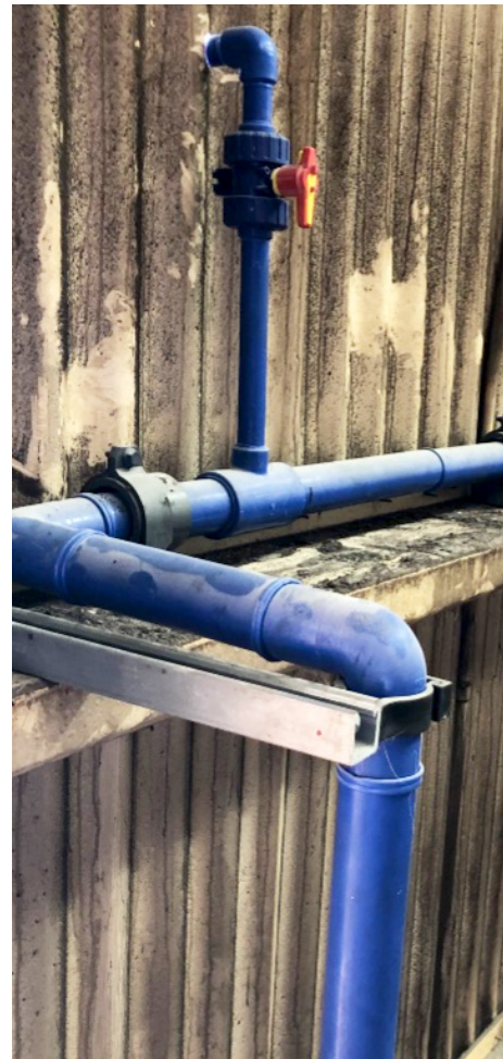
Air-Pro® at a fertilizer manufacturing facility covered in chemical dust.
