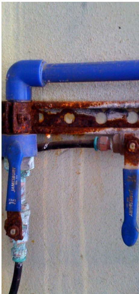
Air-Pro® at a bleach plant.
